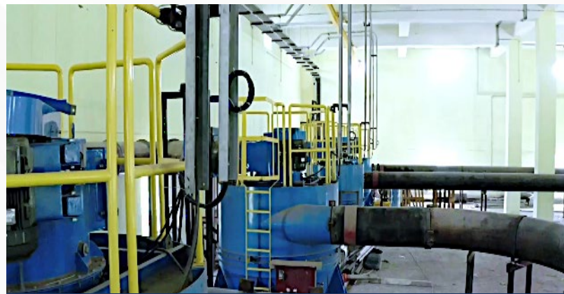
Pneumatic Waste Collection System
